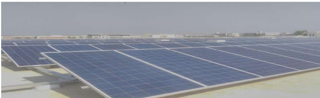
100KW Solar Power Plant Located at Rooftop of SIEM, Nashik
